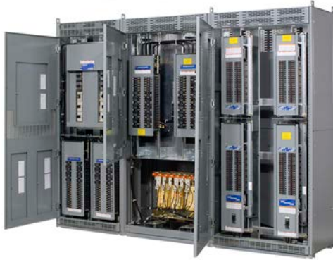
Integrated Power Center 2
