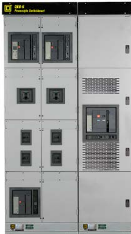
QED-6 Switchboard with MasterPact NW/NT and Powerpact H/J Circuit Breakers (Class 2746)
